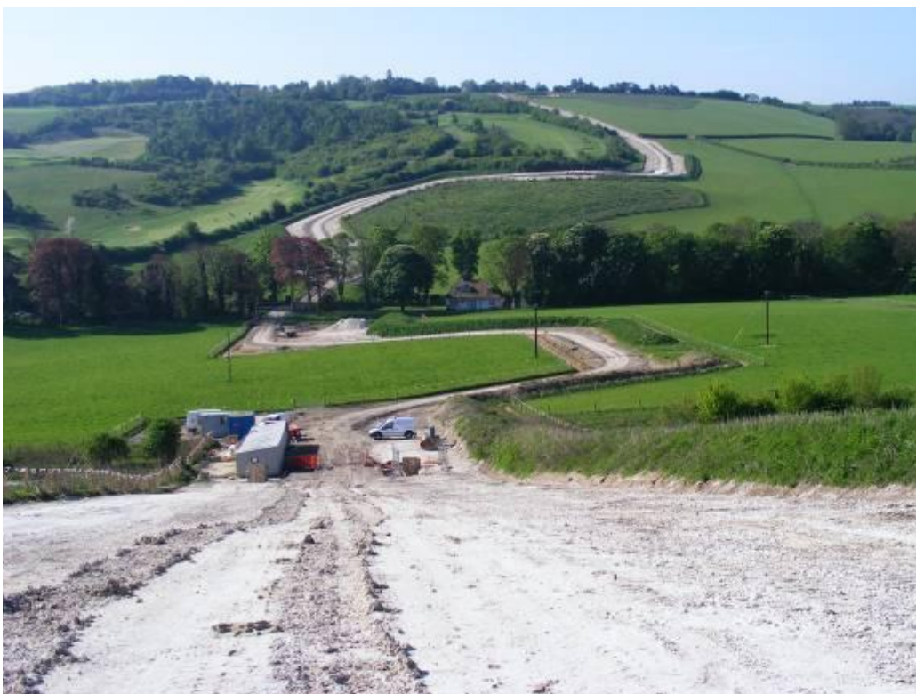
Figure 35 – 400kV cable swathe at the Goring Gap
